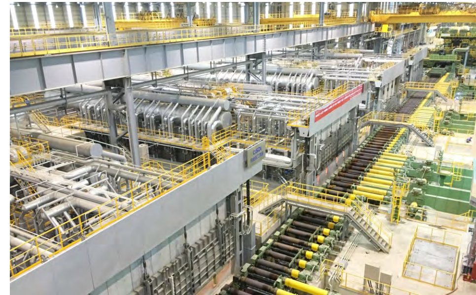
Reheating furnaces at Formosa Ha Tinh Steel in Vietnam
