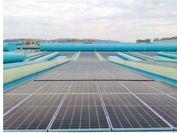
A view of the distributed roof photovoltaic power generation plant at Baowu Aluminium
